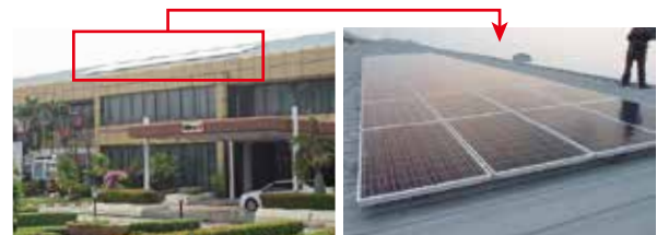
Solar panels installed on the factory roof
