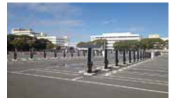
Regular charging station at the employee parking in Okazaki district
