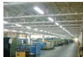
Production line LED lightings have been introduced
