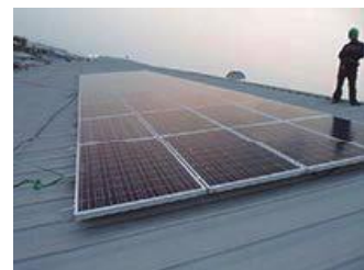
Photovoltaic power generation panels
