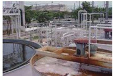
General effluent treatment facilities
