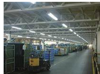
In-plant LED lighting
