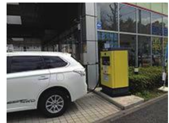
Quick charger installed in a dealer
